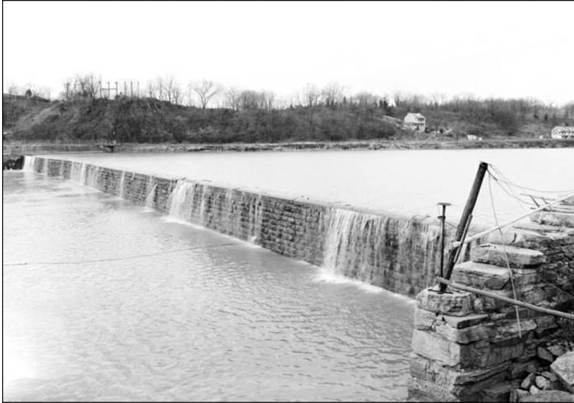
Fig. 10. Chesapeake and Ohio Canal, Dam 5, Williamsport vicinity, Maryland, c. 1860, designer unknown (Library of Congress, Prints and Photographs Division, Historic American Buildings Survey, HABS MD, 22-FOFR.V, 4-1).
