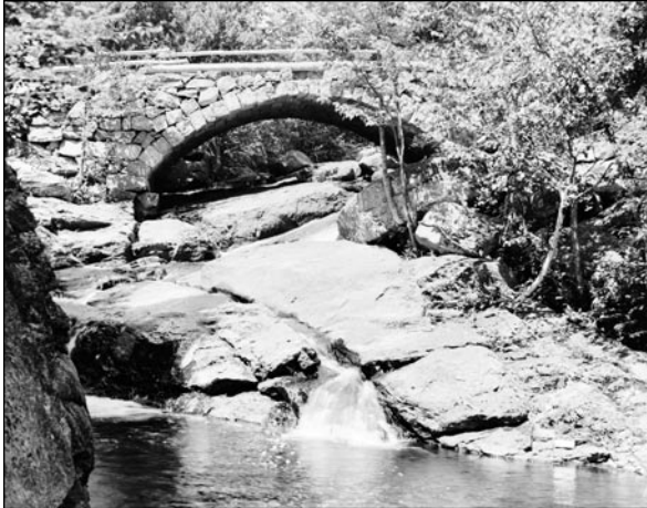
Fig. 3. Gleason Falls Dry-Laid Stone Arch Bridge, Beard Brook, Hillsborough, New Hampshire, mid-nineteenth century, designer unknown (Library of Congress, Prints and Photographs Division, Historic American Buildings Survey, HABS NH, 6-HILL.V, ID-2).
